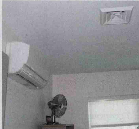
Wall-mounted units inside each apartment.
