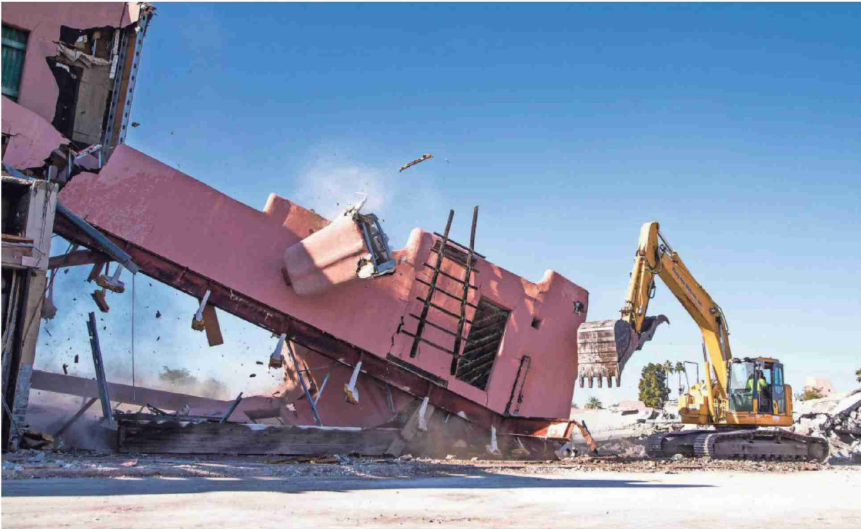
The Papago Plaza in Scottsdale is being demolished. Workers tear down parts of the buildings, Thursday. The shopping center, Scottsdale's oldest, is being replaced with a contemporary mixed-use development. TOM TINGLE/THE REPUBLIC
